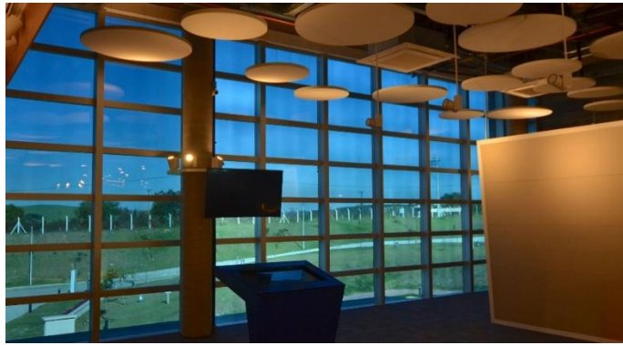
Figure 20 – Electrochromic glazing installed at Saint-Gobain Research Brazil.
