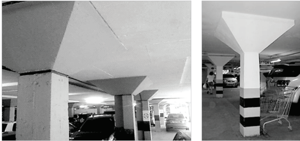
Figure 2 – Mushroom slab with a combination of drop panel and capital in a garage building in Brazil
