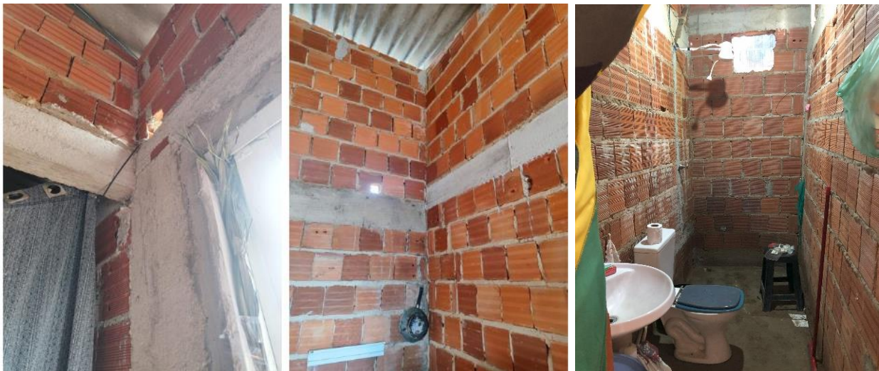
(a) Beams are not supported by columns (b) Misaligned beams (c) Misaligned beams and lack of ventilation
