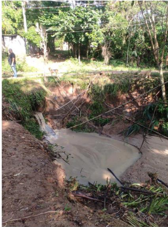
Figure 9. Discharge of stormwater from the Nova Itatiba II development into the stream of Quilombo Brotas (São Paulo State Public Prosecutor's Office, 2022, in: ACQB v. PMI, p. 223).
