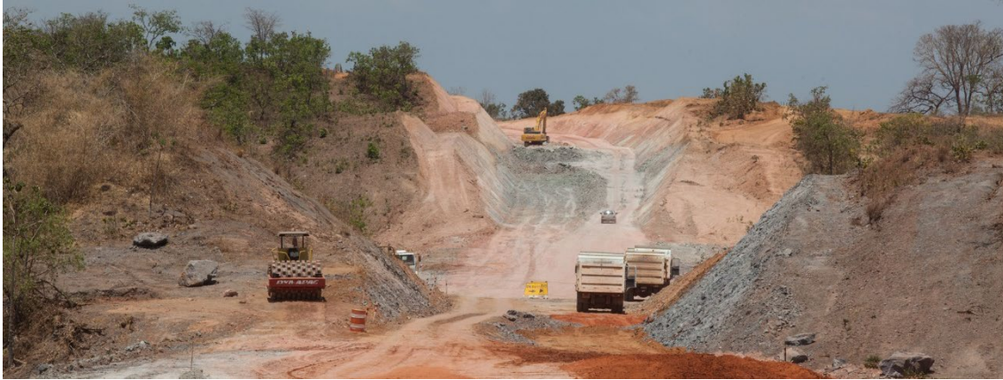
Figure 1.2. Roadworks in the southwestern part of the Araguainha impact structure, on the outer rim region, along the MT-100 state road (adapted from the SINFRA-MT – Secretaria de Estado de Infraestrutura e Logística de Mato Grosso; website: sinfra.mt.gov.br ).
