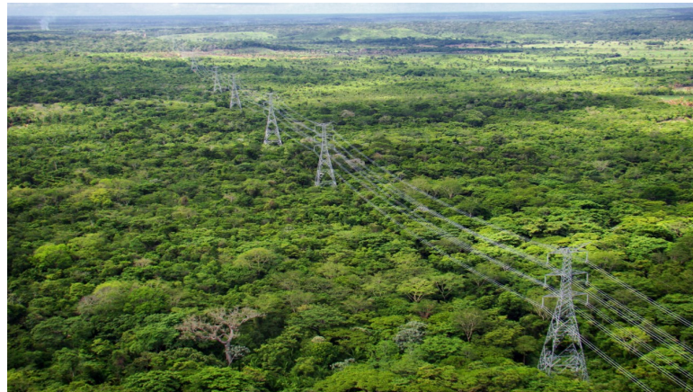
Figure 4.4: Photograph of the evaluated 500 kV double-circuit transmission line between stations Silves and Oriximiná.
