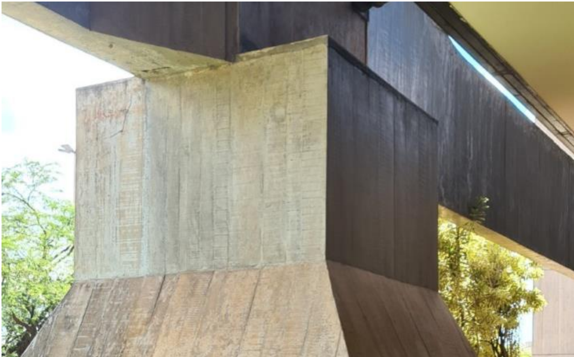
Figure 14 – Recovery and reinforcement carried out in the P4A pillar, after 15 years of execution.
