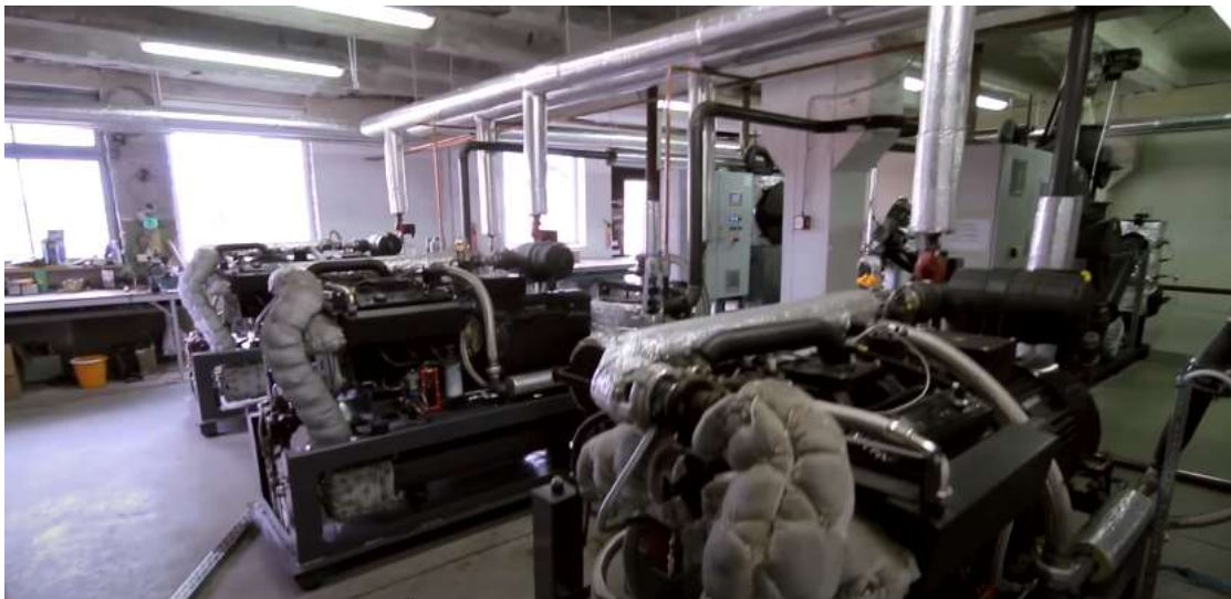
Figure 8 – Spanner Re 2 GmbH CHP plant located in Valka, Latvia.
