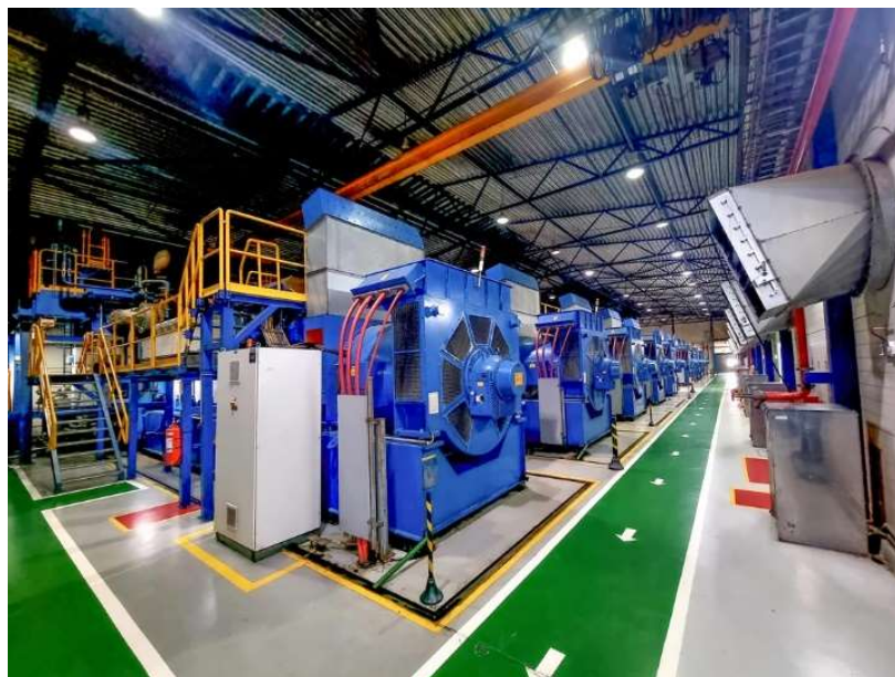
Figure 5 – Wärtsila 20V24SG gas generator sets with a total combined output of 204 MW in thermoelectric powerplant UTE-LORM, located in State of Espírito Santo – Brazil.
