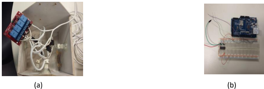
Figure 5. (a) Prototype from above model house, and (b) Automation control centre composed of an Arduino-Mega board and an Ethernet
