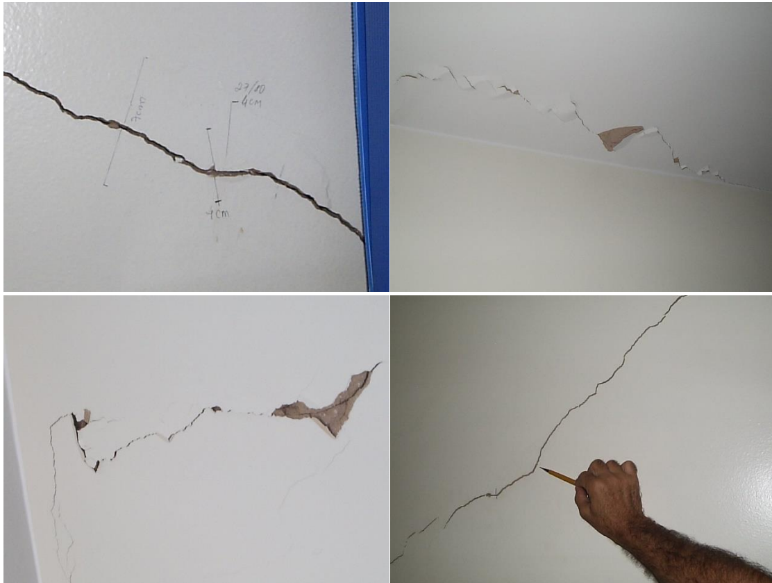
Figure 2 – Cracks and fissures observed in visual inspection in November 2005.
