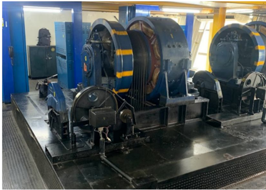
Fig. 15. Elevators with high energy-consuming electric motors
